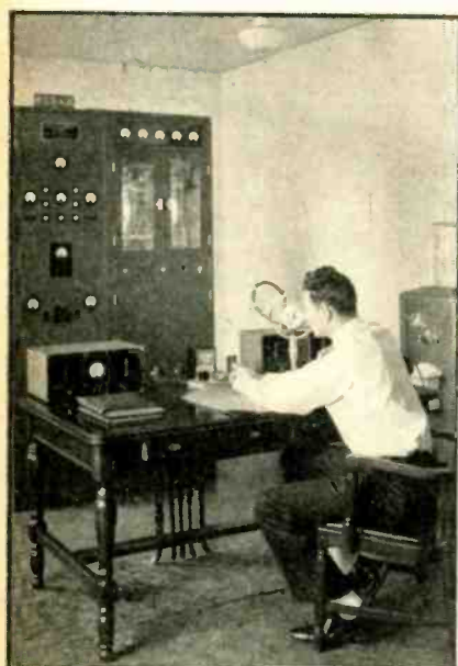
In 1934 this 50-watt u-f transmitter with 500-watt amplifier was installed by W. E. in the National Newark & Essex Bank Building
